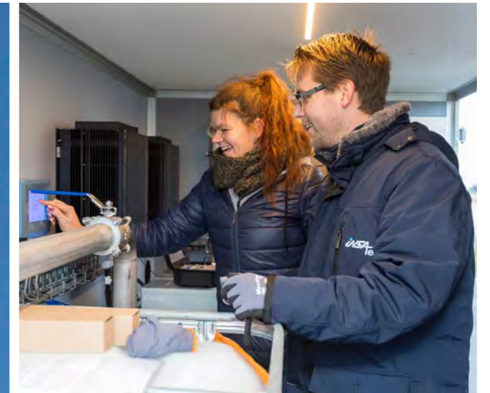
Insatech’s self-developed water purification system RemUVe ensures that drinking water is of high quality.
